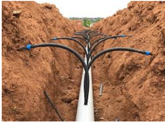
Figure 6. Underground irrigation system (URL-4)
